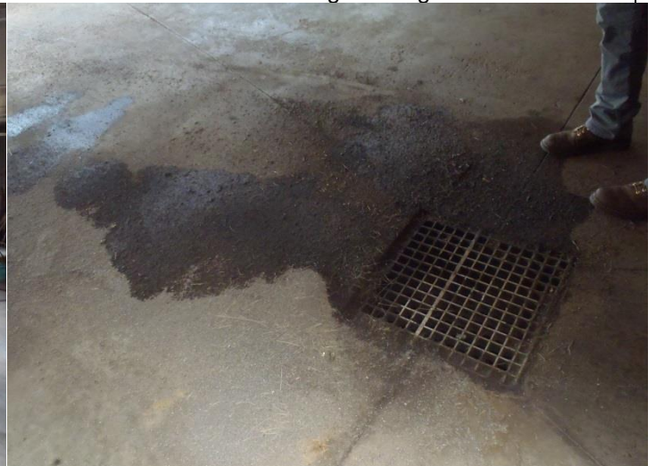
Garage Floor Drain
